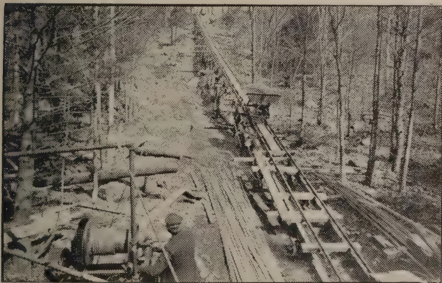
RAILWAY USED TO HAUL MATERIAL UP TO NEW STANDPIPE ON MOSES HILL Courtesy Christian Science Monitor
